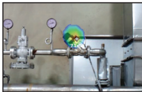
Compressed Air Leak on an Isolation Valve
